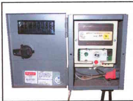
ELECTRONIC TEMPERATURE CONTROL IS USED TO KEEP THE TP CAN OIL/WATER AT BEST SEPARATION TEMPERATURE
